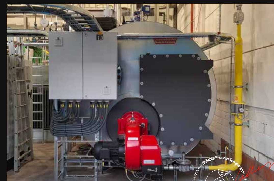
Hybrid steam boiler - 6.3 t/h
